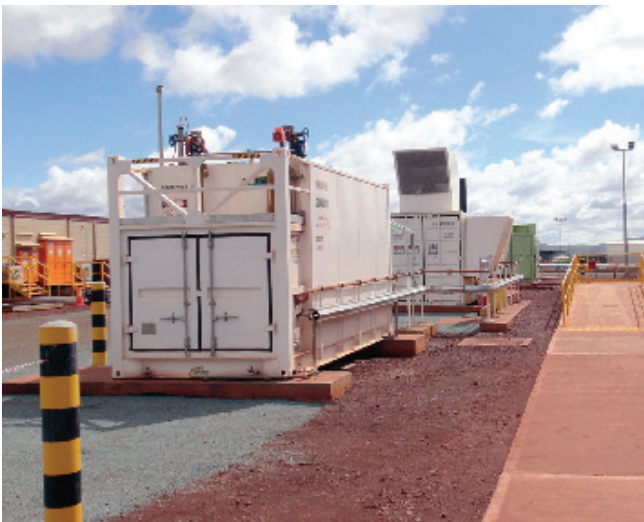
Portable Energy Refuelling
